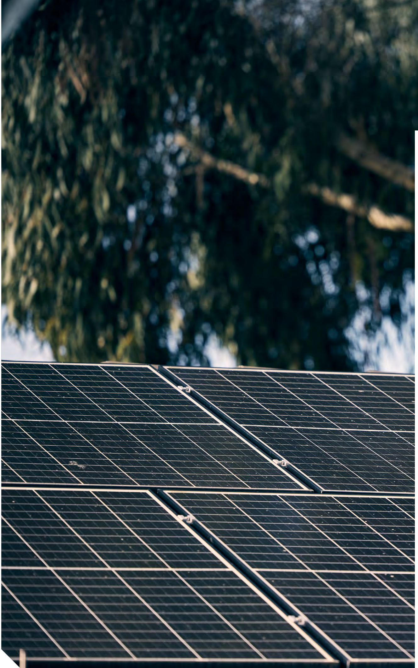
IV | Solar panel on a roof in Adelaide
