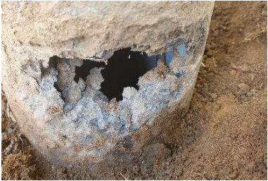
Extreme Hole in the column
