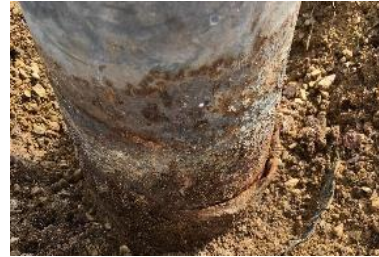
High General corrosion
