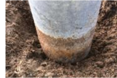
Moderate Minor corrosion
