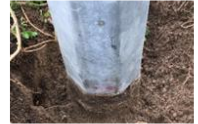
Low Signs of corrosion
