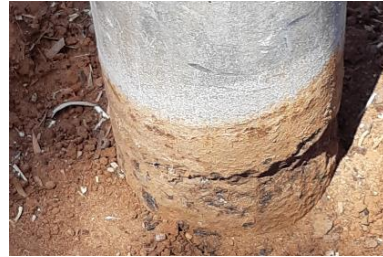
Very High Significant deteriorations and corrosion
