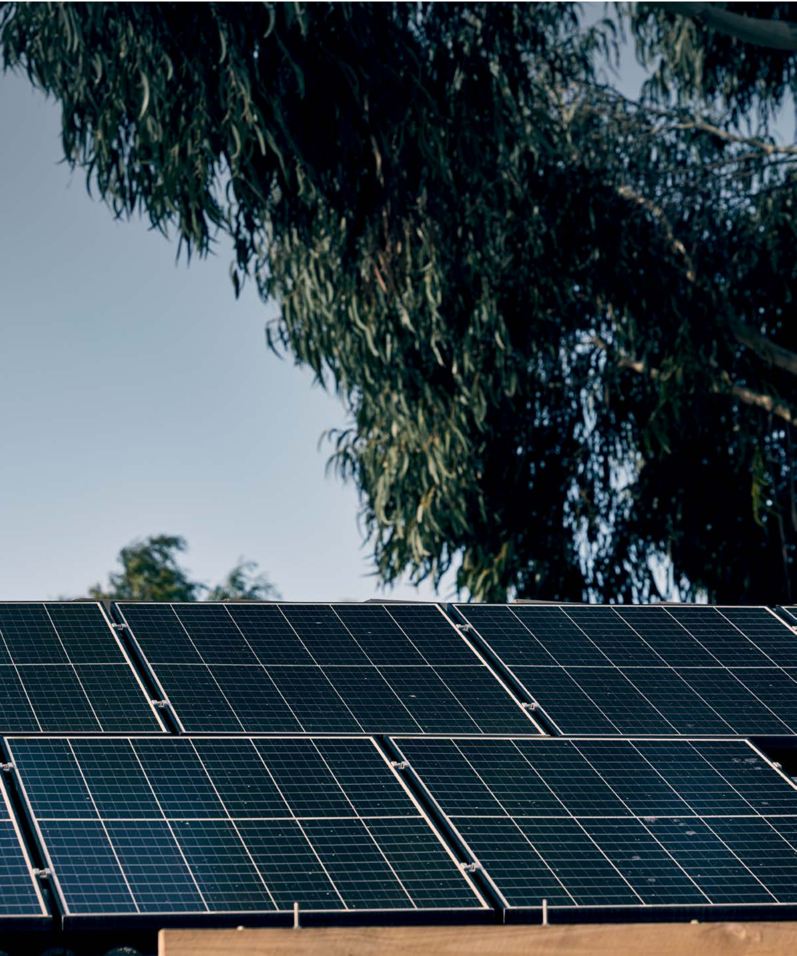
Solar panels on the roof of Andrew and Jessica’s home
