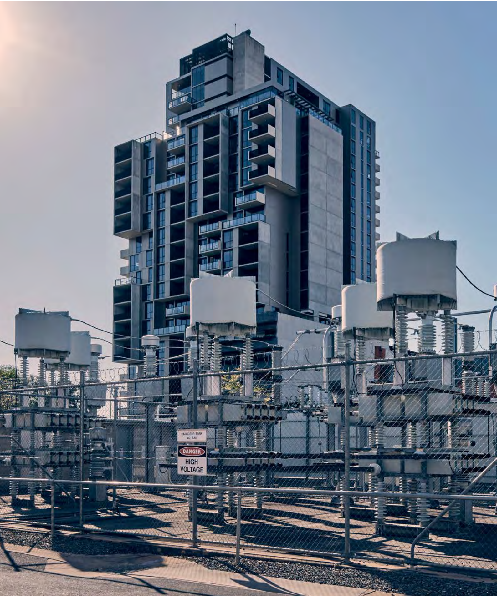
Whitmore Square Substation Central Business District
