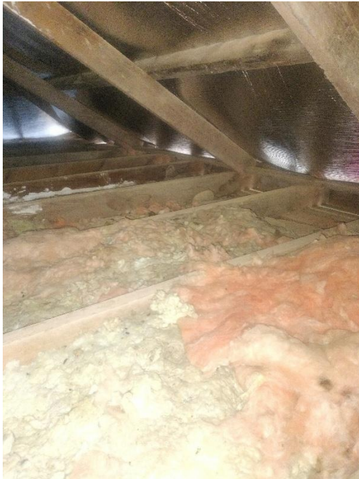
Figure 168: this house by comparison has gaps, is patchy and is not deep. It has degraded over time with animals and weather. It will not be working as it should.
