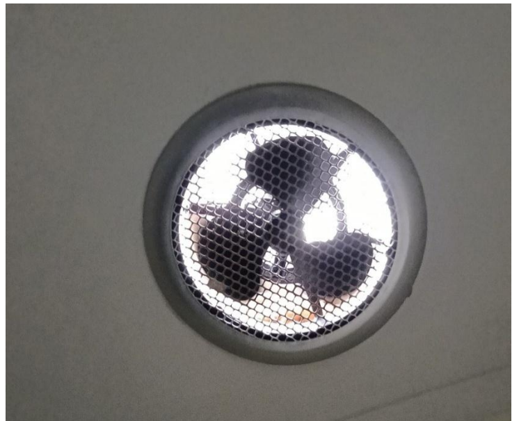
Figure 6: This fan in a bathroom does not seal itself when off, you can see directly through. This will be an area where you lose heat in winter and gain it in summer.
