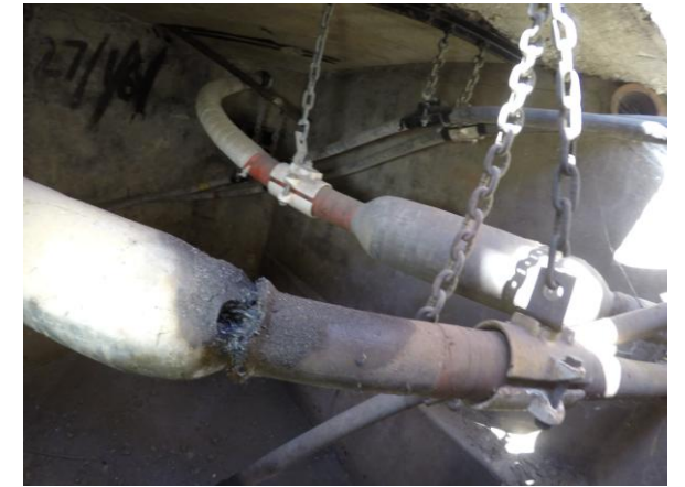
High risk/weeping joints
