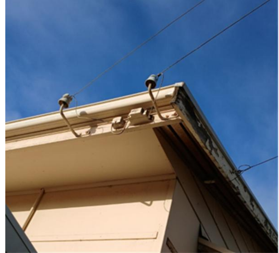
Typical Open Wire Service Connection Point
